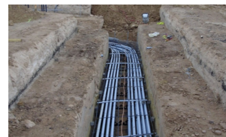
Underground Light Fitting
